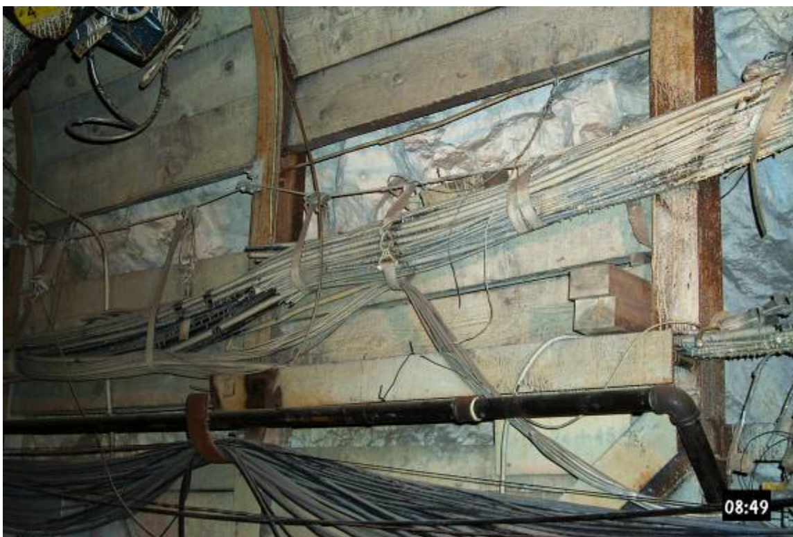
Figure 4-7. Abandoned electrical wiring scheduled for removal.
