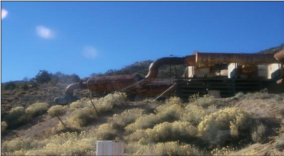
Figure 4-1. Dual 300-hp Sutorbilt Ventilation Fans.
