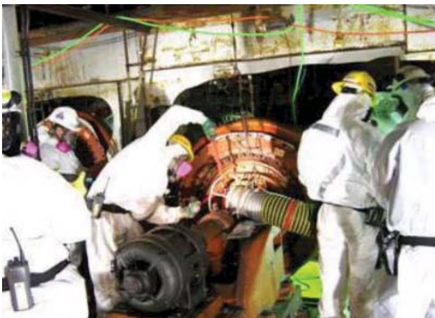
High Risk Equipment Compressor Seal Exhaust Lines are Cut and Isolated
