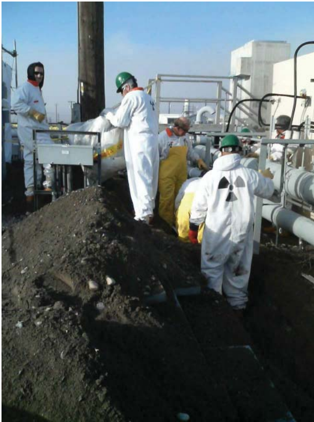
Preparing To Replace a Hose-in-Hose Waste Transfer Pipeline in SY Tank Farm
