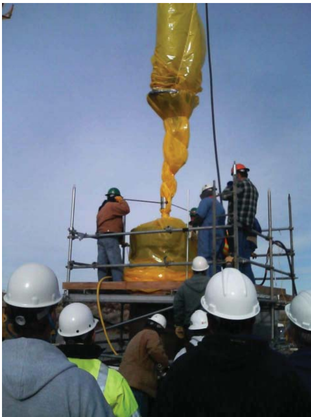
Mockup Training To Remove Slurry Distribution in Tank AY-102 and To Install a Waste Transfer Pump
