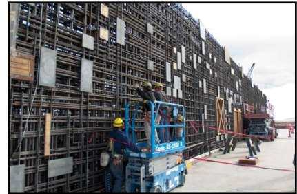
Employees tie rebar on the fifth lift walls at the Pretreatment Facility.
