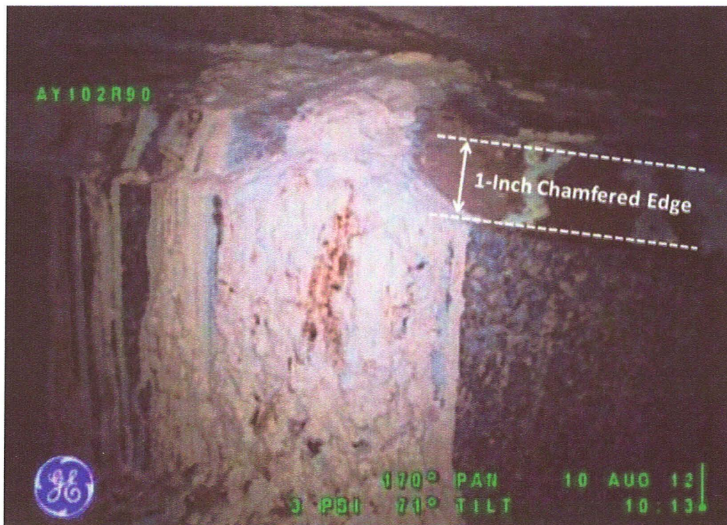
Figure 4. Close-up of dried tank waste in the refractory slot (from RPP-ASMT-53793).
