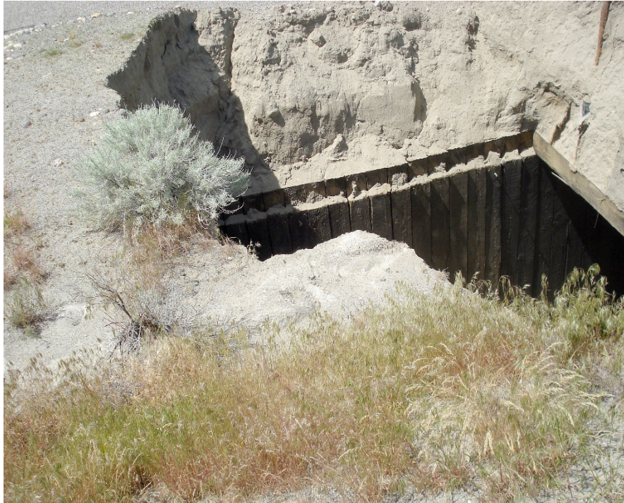
Partial Collapse of PUREX Tunnel #1
