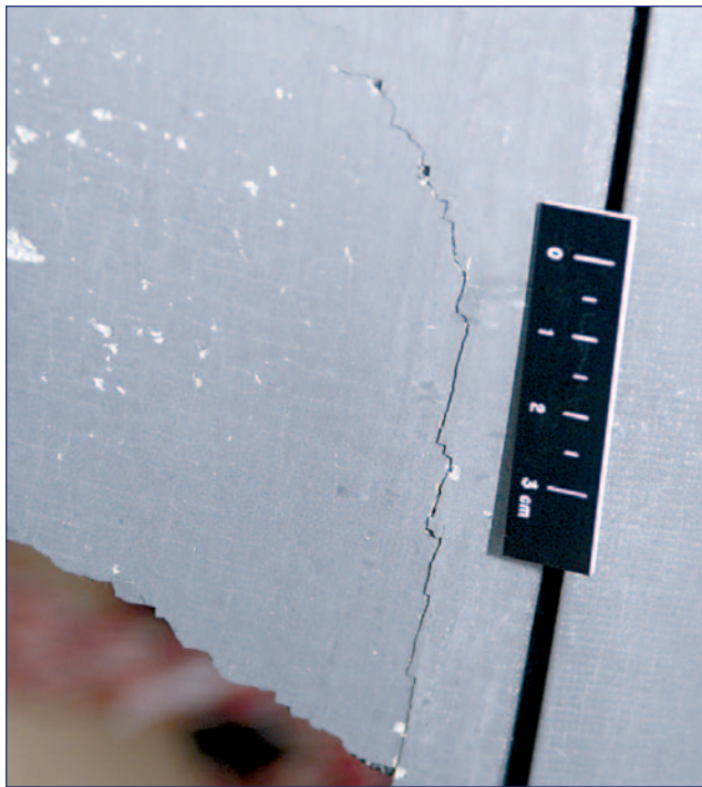
Figure 3.8-10. Numerous cracks were also noted in RCC Panel 8.
